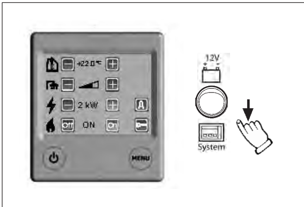
The boiler's control panel
