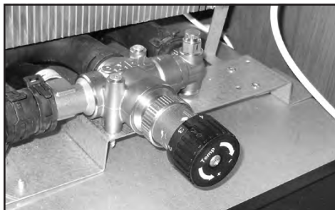
AGS II Pro floor heating is recognisable from the shunt valve by the boiler.
