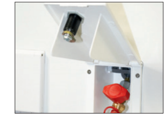
Exterior gas outlet
