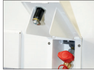
Exterior gas outlet
