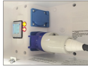
Electricity meter in the electrical box
