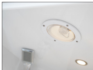
Ventilator in de badkamer (TDL, 780 DGLE)
