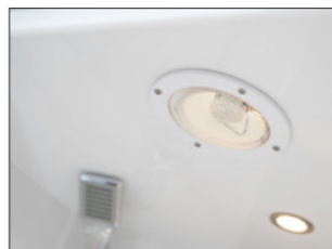
Ventilator i brusebad (TDL)
