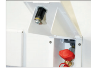
Exterior gas outlet
