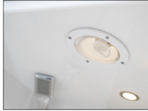
Ventilator in de badkamer (TDL, 780 DGLE)
